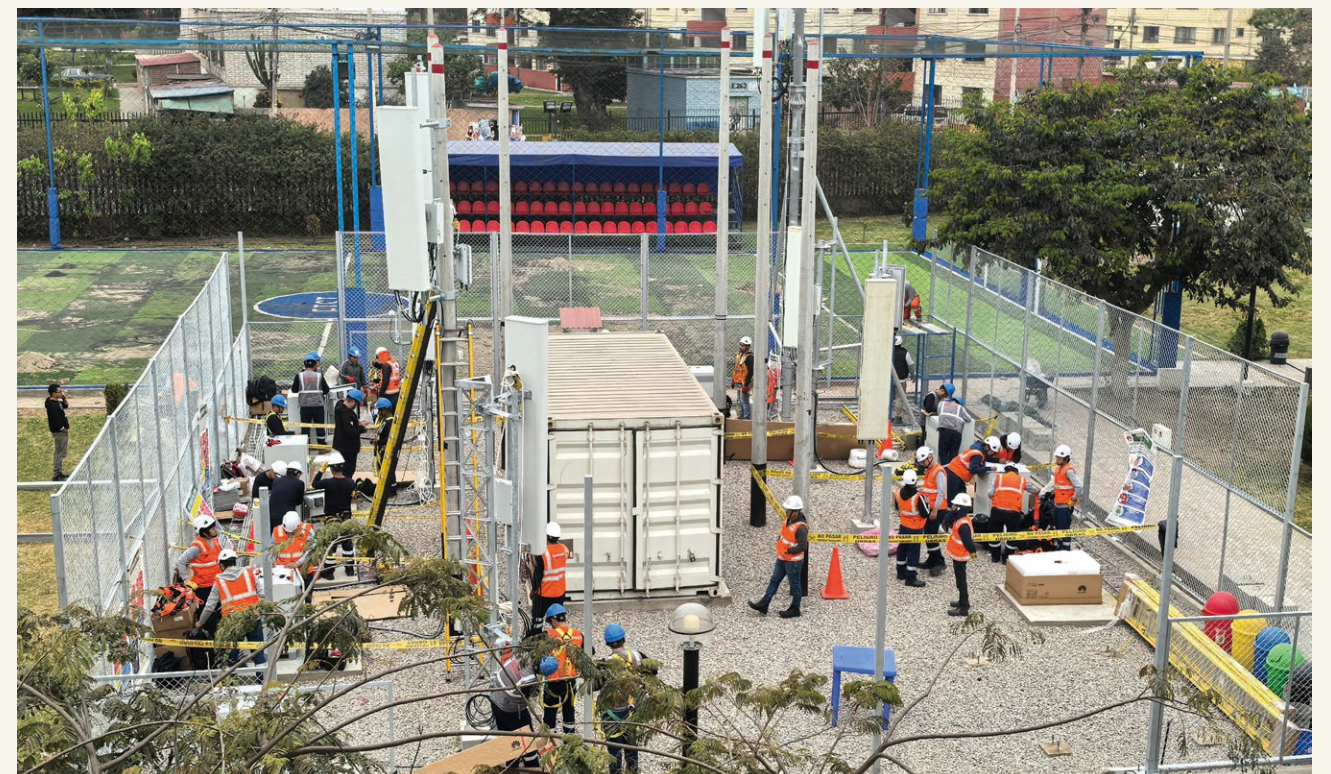
| EHS training and practice at a hardware installation site
